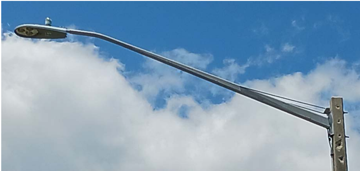
Aluminum Arm on Concrete pole
