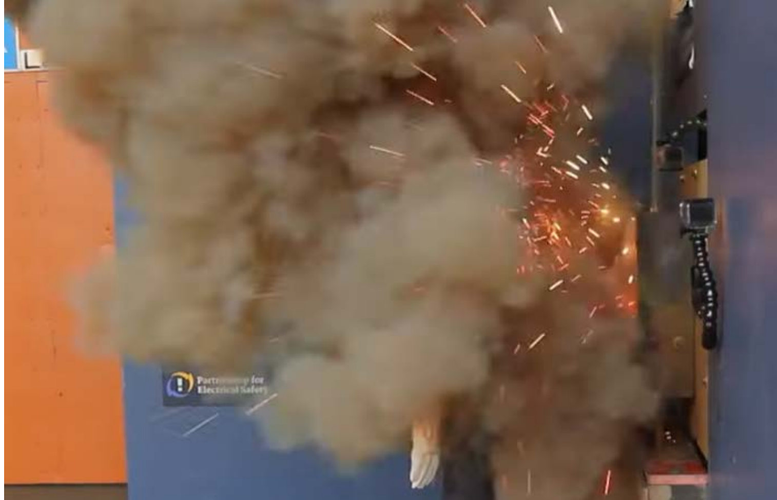
Occupational Safety and Health Administration (OSHA), U.S. Department of Labor. "Electric-Arc Flash Hazards". Published on OSHA website, embed at: https://www.youtube.com/watch?v=GyNqmcqKZ-8 . Public domain (U.S. government work), with some third-party testing footage courtesy of KEMA Laboratories & Partnership for Electrical Safety.
